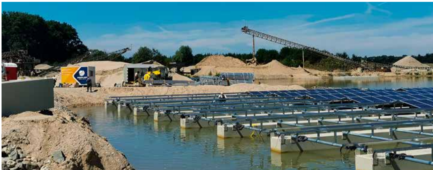
Fig. 6 – 750 kW floating PV on a dredging lake of a gravel pit (Photo: © Energieagentur.NRW / Rheinland Solar).
