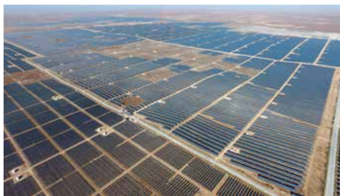
Fig. 4 - Ningxia 2 GW PV project (Photo: SUNGROW).
