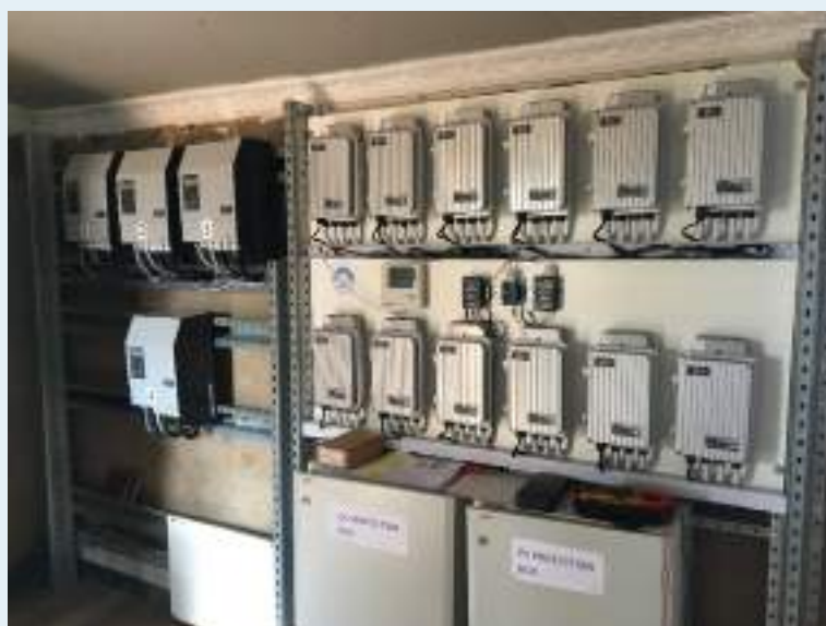
Figure 39 Inverters and MPPT solar controllers
